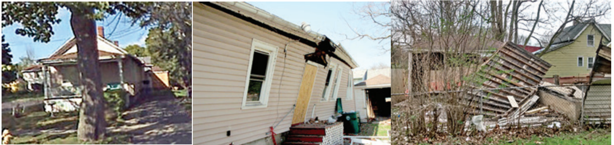
Before, during and after Isaiah 61 tackled the renovation of a home on Centre Ave. Failure to put proper support beams in the attic of this home caused it to collapse.
