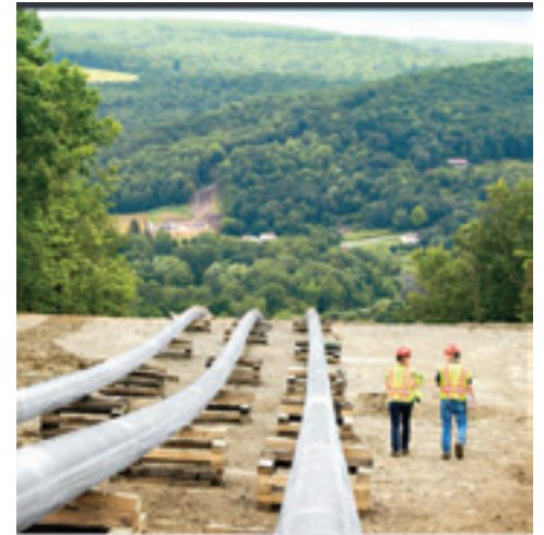
The cover of National Fuel Gas' 2015 annual report shows a pipeline running directly into a scenic rural town and two helmeted workers walking along it for perspective.
