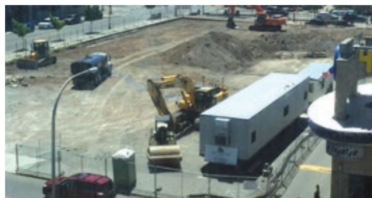
Not much activity at Hamister hotel site...officials mum so far on formal groundbreaking
