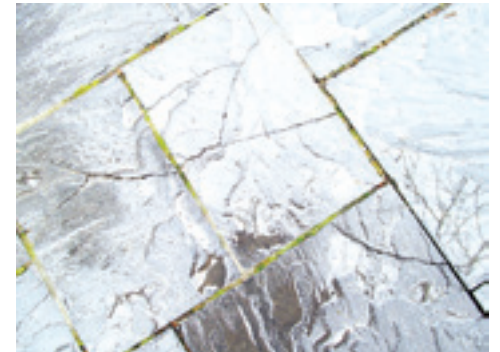
Three adjacent pavers in the Niagara Falls State Park, all exhibiting cracks.
