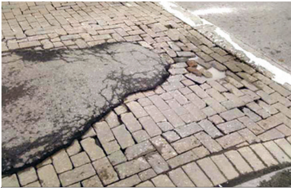
A gob of blacktop was the sloppy repair strategy for a cobblestone crosswalk at Third and Niagara. Funded by USA Niagara and the city, ten years later the collapsing cobblestone of the "Revitalization Initiative" is scandalous, stark evidence of yet another "economic development" boondoggle .
