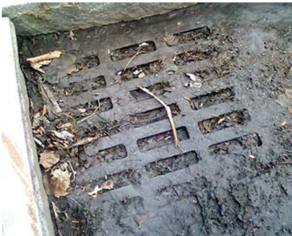
A storm drain on Third Street plugged with refuse and muck graces the city's vaunted tourism district.
